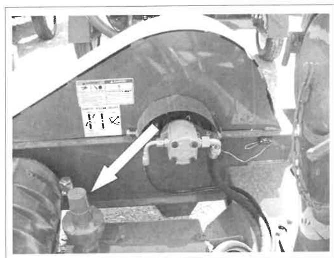
Fig. 5-13 Pressure Relief Valve.
