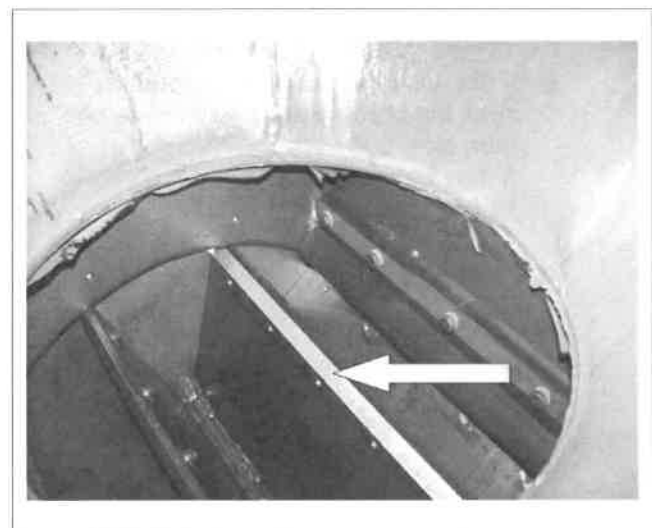
Fig. 5-29 Checking Tip Clearance Through The Access Door.
